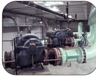
Process Water Pipeline Systems
